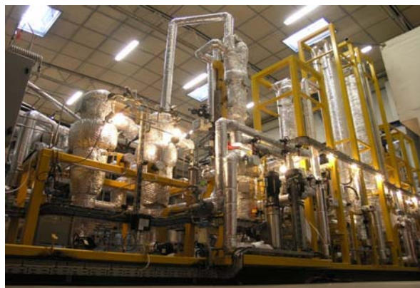
Figure 1: Picture of the pilot plant at Fortum's CHP Plant in Stockholm
